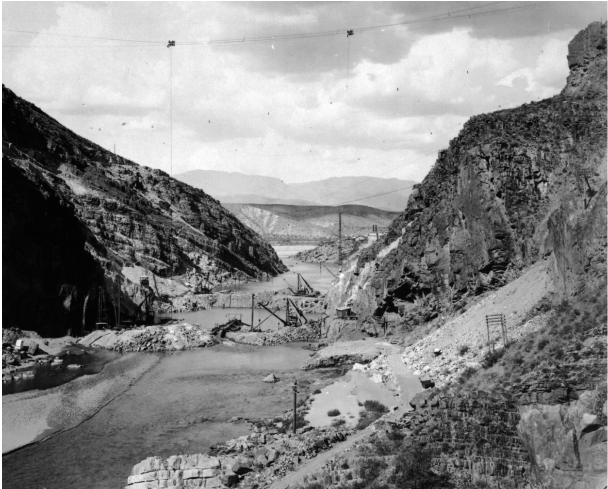
Figure 44: Roosevelt Dam under construction, July 27, 1906. There were no objections by navigation interests to the construction of the dam found in any Reclamation Service records. Source: Records of the U.S. Bureau of Reclamation, U.S. National Archives branch, Denver, Colorado.
