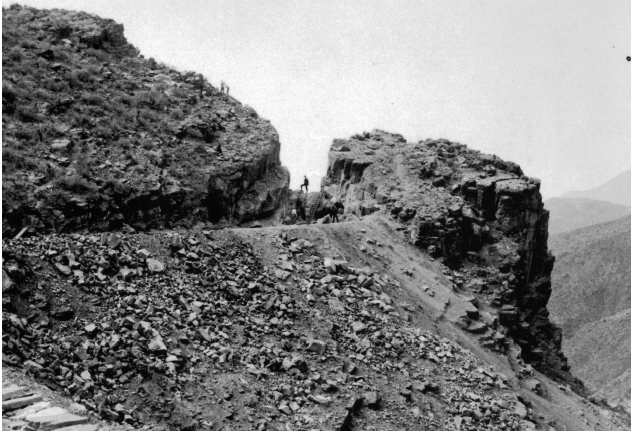
Figure 46: Work on excavating notch on Roosevelt Road above Roosevelt Dam site, ca. 1906. Source: Records of the U.S. Bureau of Reclamation, U.S. National Archives branch, Denver Colorado.
