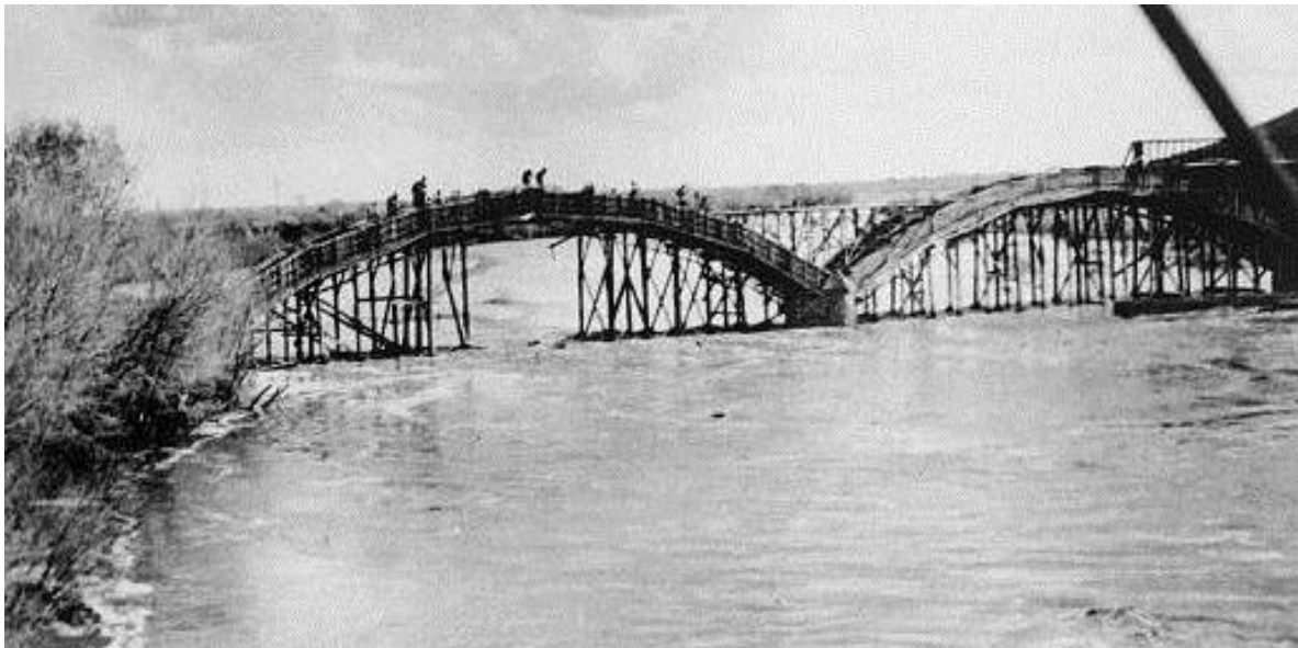
Figure 76: Ash Avenue Bridge between Phoenix and Tempe under construction using convict labor, 1912. Note heavy flow in Salt River. Source: U.S. Library of Congress, Washington, D.C.
