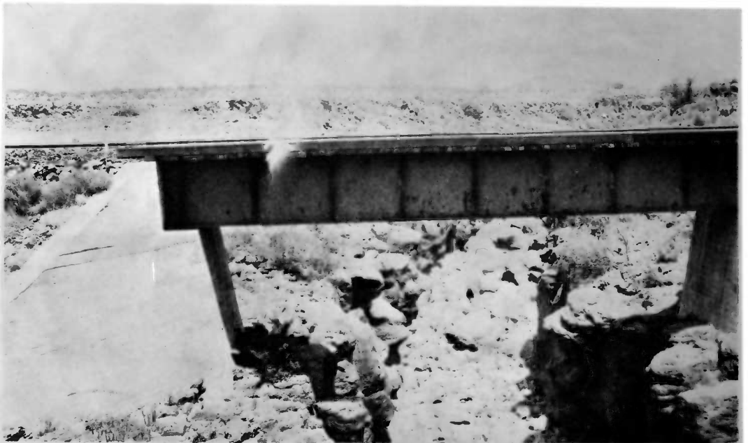
S.F.R.R. Bridge Over Head of Verde River Looking East from Highway, July 25, 1940
