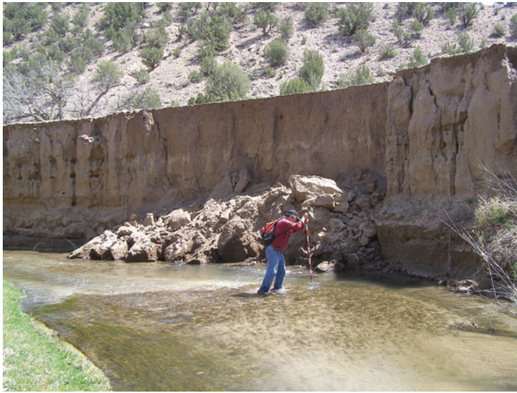
Figure 4.7 —Vertical streambank collapse as a source of sediment in the UVR. (Photo by Daniel G. Neary.)
