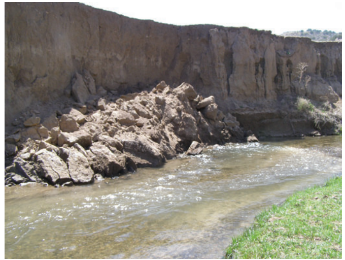
Figure 5.4 —Unconsolidated Holocene river-deposited sediments along the UVR channel near Burnt Ranch. (Photo by Daniel G. Neary.)
