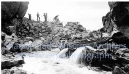
Construction of Sullivan Lake Dam in 1935. The base flow that is diverted around the construction area is mostly from tributary streams (Qmf and Qqa). A very rough estimate is 5cfs.
