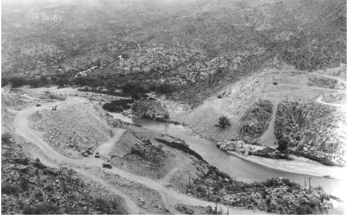
Figure 41: Bartlett dam site, 1936. Source: Records of the Bureau of Reclamation, U.S. National Archives Branch, Denver, Colorado.
