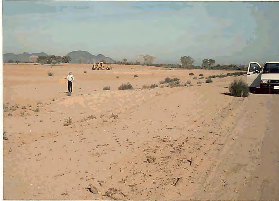
E. Looking at left overflow area from left bank of main channel.
