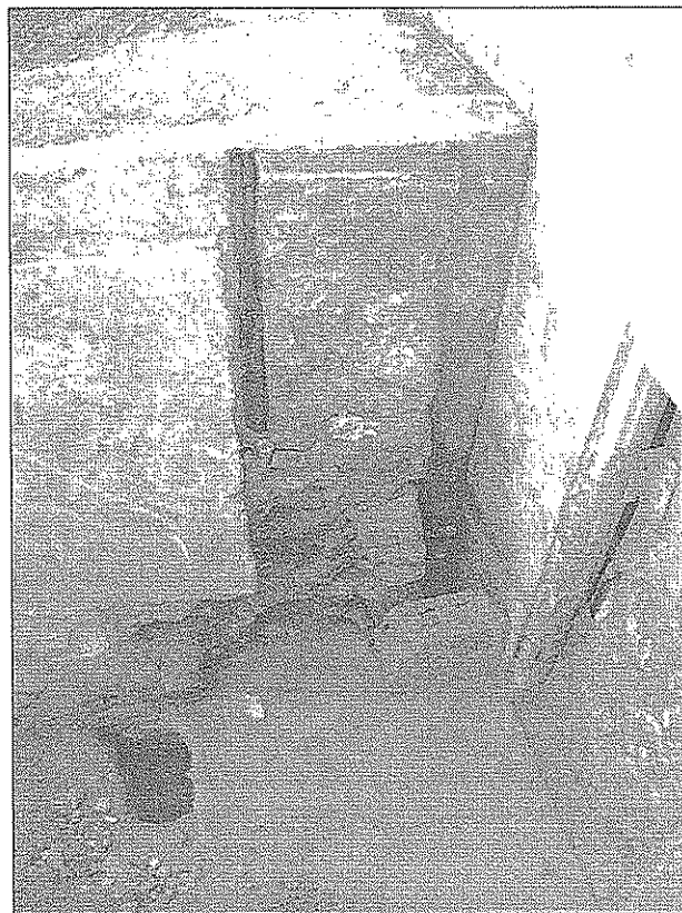
Figure 24.29. Photograph of rock support wall Feature 14 showing what may be a junction with the original adobe flour mill Feature 53 (Wall Segment 6, AZ U:9:278[ASM]), facing south.
