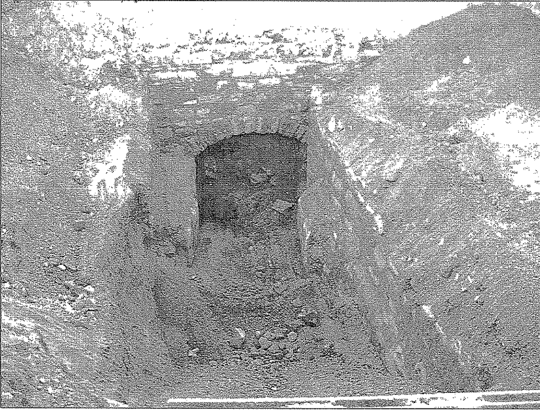
Figure 24.7. Photograph of intact rock-walled western retaining wall Feature 7 (tail race), Hayden Ditch site (AZ U:9:189[ASM]), exposed in Phase 2 backhoe trench U2139, facing south. Note the turnout gate (Subfeature 7.02) remnants in front of the stone arch (Feature 67; AZ U:9:278[ASM]).
