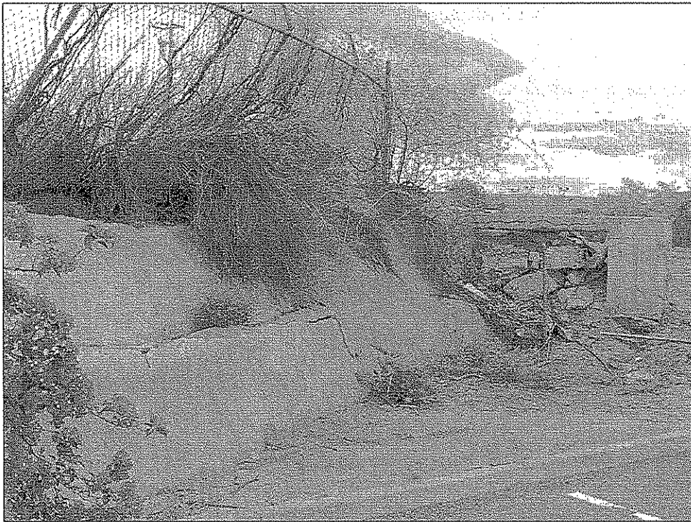
Figure 24.58. Photograph of the southern terminus of gunnite berm Feature 4 at check/drop Feature 3, Hayden Ditch site (AZ U:9:189[ASM]), facing southeast.
