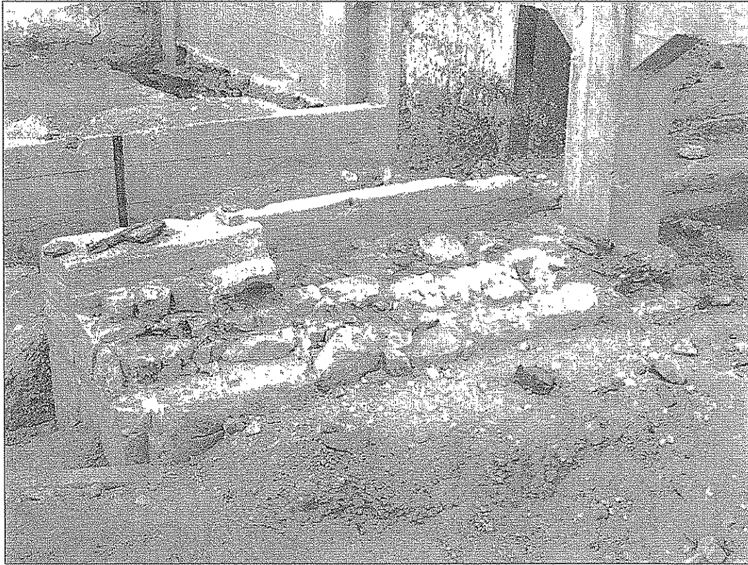
Figure 24.21. Photograph of Subfeature 11.02, a rock-lined junction dividing wall, Hayden Ditch site (AZ U:9:189[ASM]), facing northwest.
