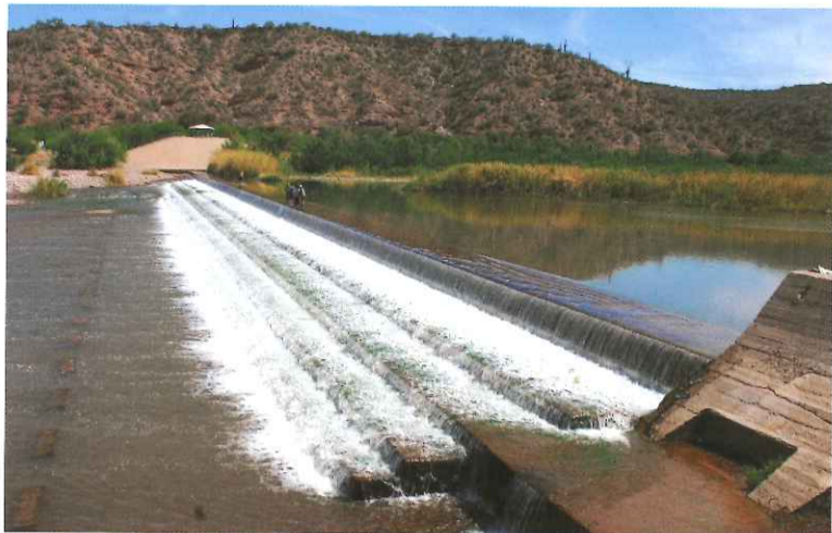
This diversion dam is located 0.8 miles past the Highway 288 river access and is a significant hazard at high water.
