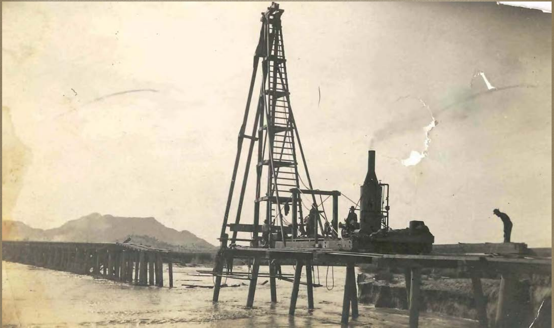
Workers driving pilings to repair the railroad bridge damaged in 1905 by the Gila River flood. Source: Arizona Historical Society, Tucson, Arizona.
