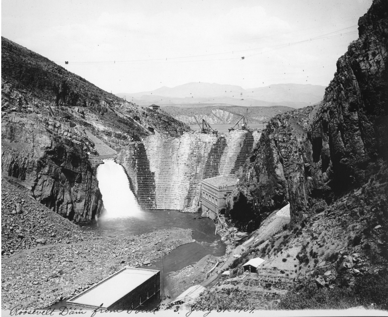
Figure 26: Roosevelt Dam under construction, July 31, 1909. Source: Records of the Bureau of Reclamation, U.S. National Archives Branch, Rocky Mountain Region, Denver, Colorado.
