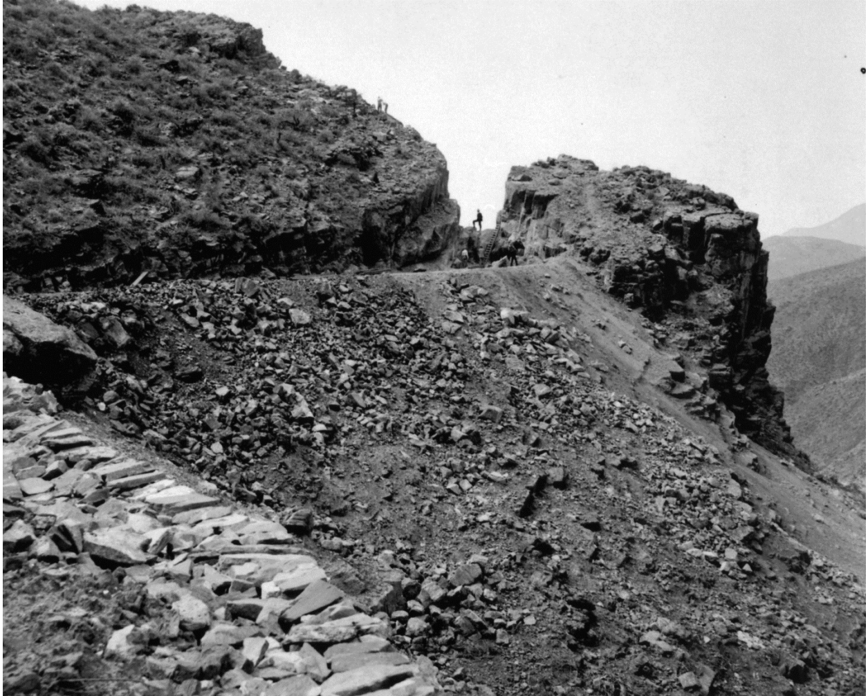
Figure 28: Construction of high-line wagon road directly above Roosevelt Dam site, March 29, 1905. Source: Records of the Bureau of Reclamation, U.S. National Archives Branch, Rocky Mountain Region, Denver, Colorado.
