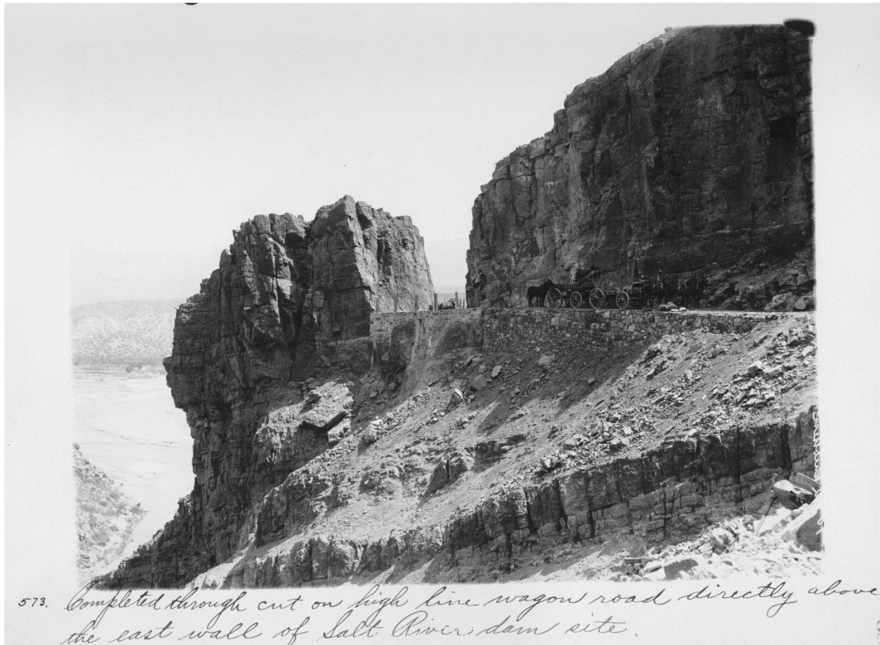
Figure 30: Completed cut for wagon road above Roosevelt Dam site, circa 1906-1907. Source: Records of the Bureau of Reclamation, U.S. National Archives Branch, Rocky Mountain Region, Denver, Colorado.
