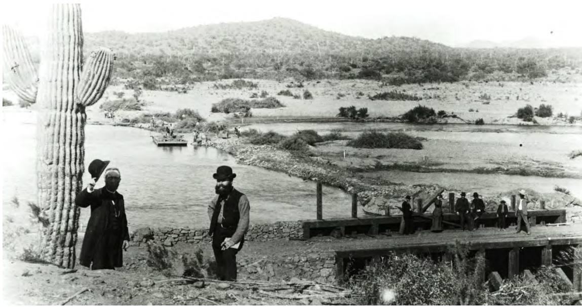
Figure 82: Arizona Canal construction (or repair), 1885, with skiff in background. Note headgate in foreground, and immediately above the group of people on the headgate is one channel of the Salt River (blocked by rocks and dirt). The remaining channel above is still open, but workers on the skiff appear to be filling that channel to divert all of the Salt River into the headgate. Source: Special Collection Collections, Arizona State University, Tempe, Arizona.
