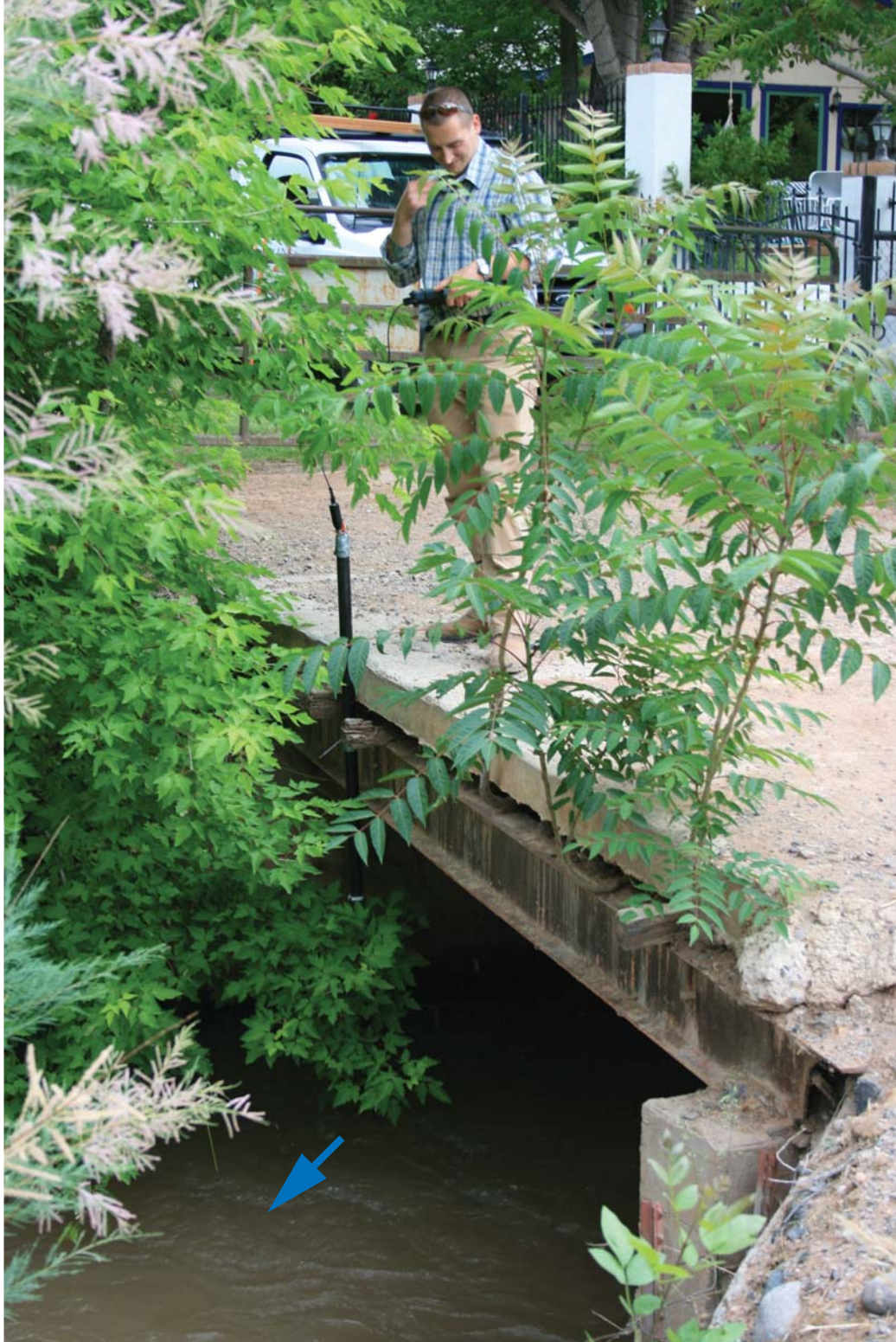
Figure 37 - Pressure transducer installed at Verde Ditch head gate prior to high-flow displacement, Camp Verde, central Arizona. Instrument was recovered after August 2009 floods and relocated to river left side of structure. Blue arrow indicates flow direction.
