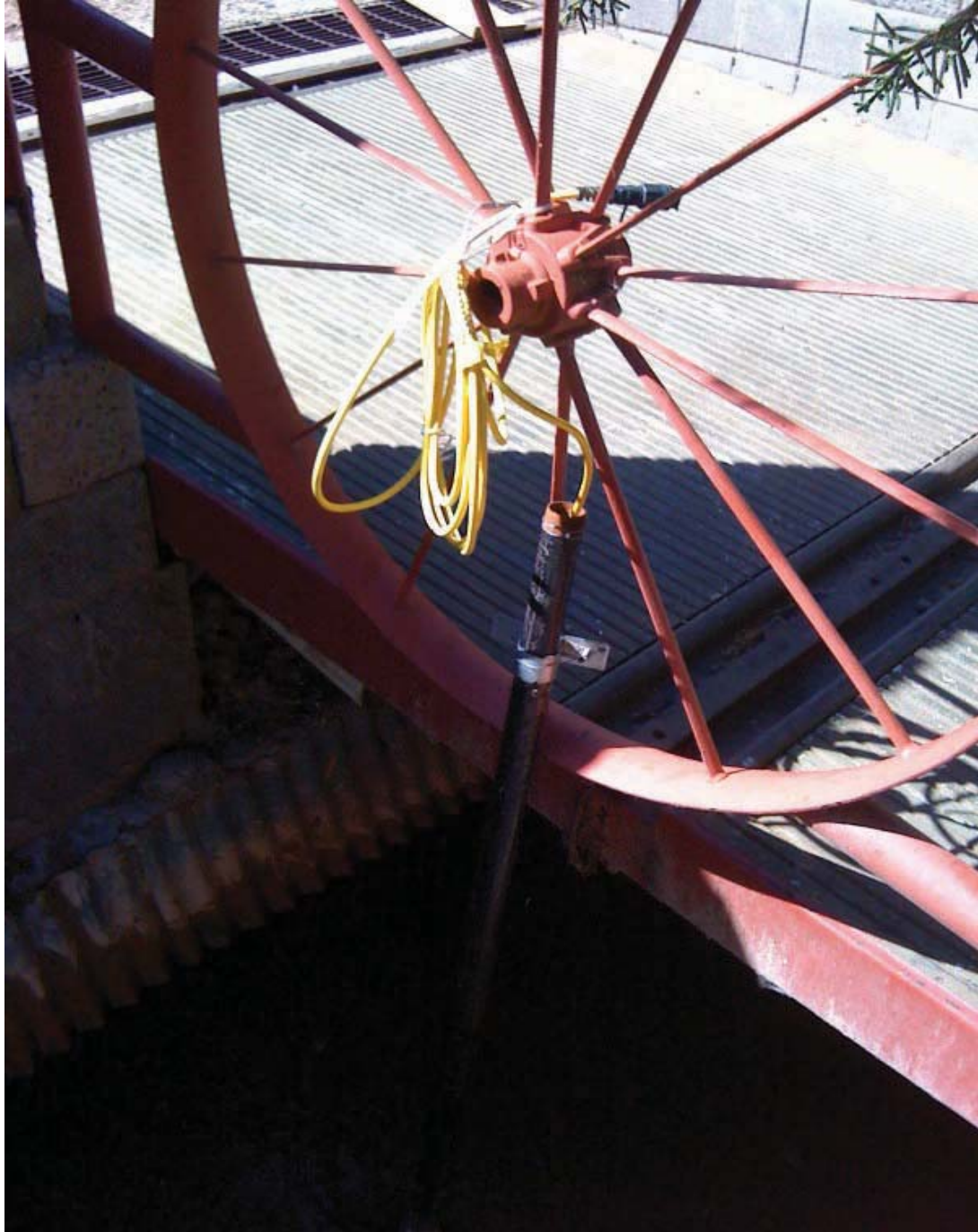
Figure 32 - Pressure transducer installed at Eureka Ditch return flow, Camp Verde, central Arizona. Shortly after this location, flow is returned to Beaver Creek.
