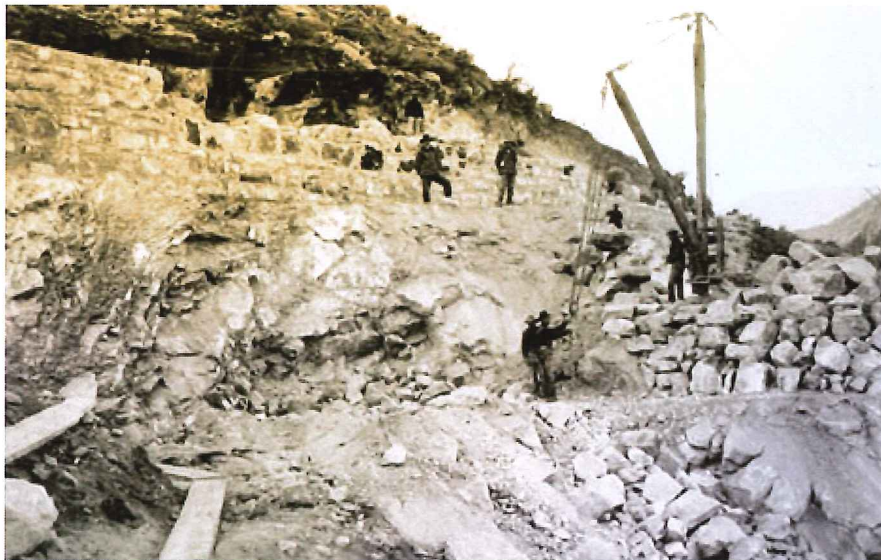
Cement was made at the dam site to save money by avoiding the cost of hauling it from Phoenix. In this 1904 photograph, Lubken captures construction workers building the cement plant. (Reclamation photograph)
