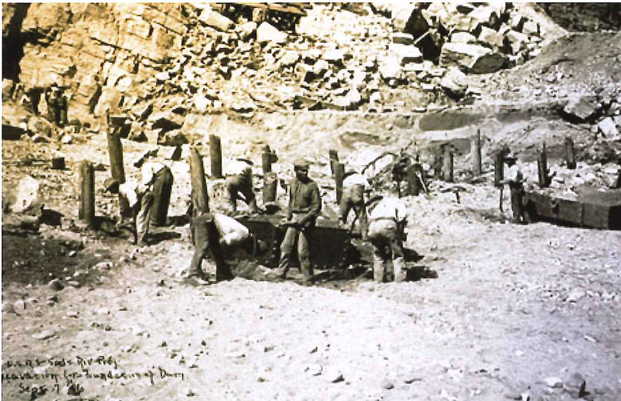
Workers from Arizona Territory—Black, Indian, Mexican, and Anglo—were joined by hundreds of other workers from numerous ethnic backgrounds from across the United States to work on Roosevelt Dam. Here they are pictured excavating the foundation for the dam, 1906. (Reclamation photograph)
