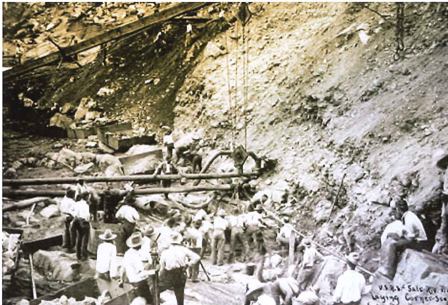
On September 20, 1906 workers ease the cornerstone of the dam into place. (Reclamation photograph)
