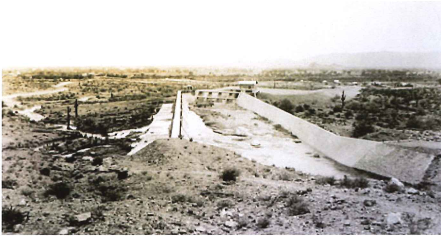
The purpose of the forebay was to hold a steady head of water for power generation. More importantly, it allowed the water to settle and drop its silt and sand to the bottom of the forebay where could be flushed out as necessary, 1914. (Reclamation photograph)
