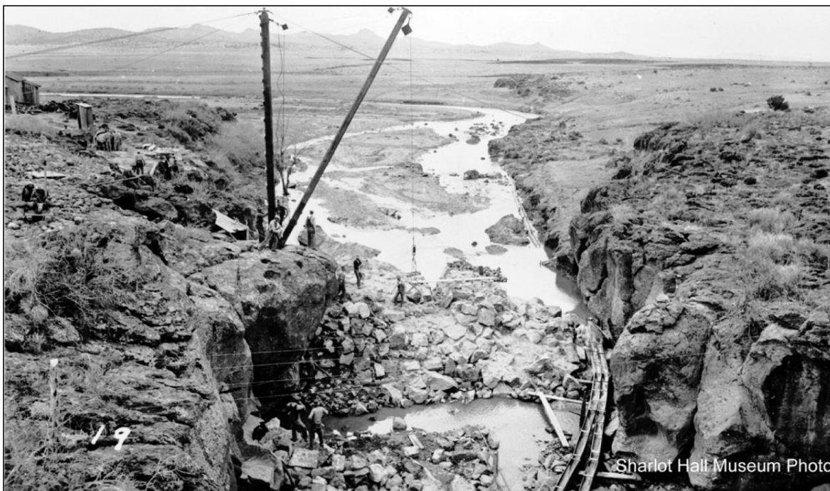
Sullivan Lake Dam construction in 1935 showing base flow. Most of the base flow is from Big Chino Valley area but some is from Little Chino Valley.
