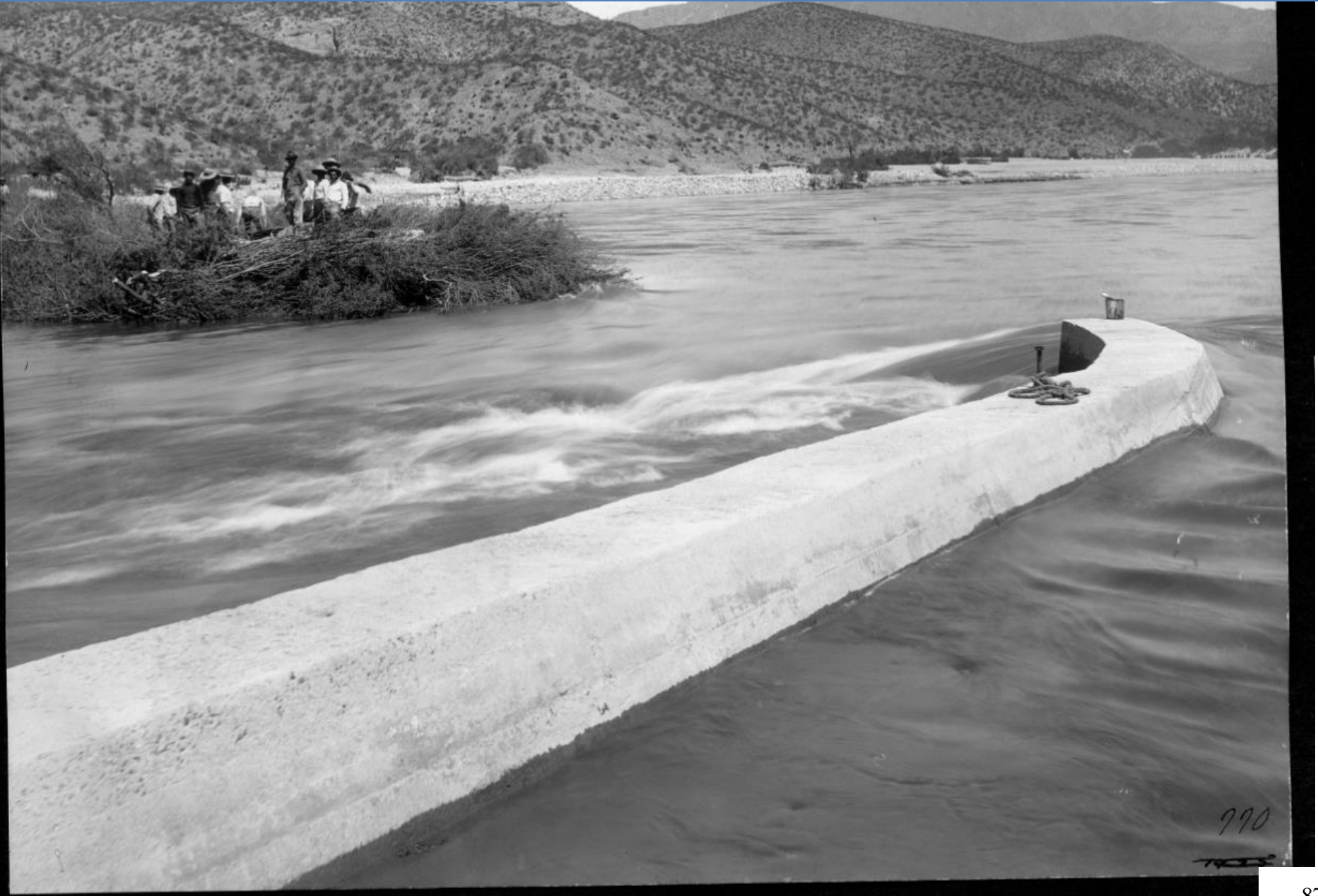
Temporary Bush Dam Being Constructed at Intake of Salt River Power Canal (Lubken), May 1, 1906
